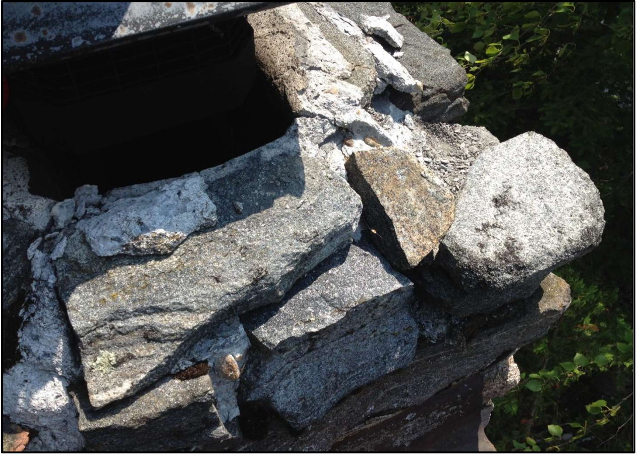
Deteriorating chimney on Little House needs repaired.
