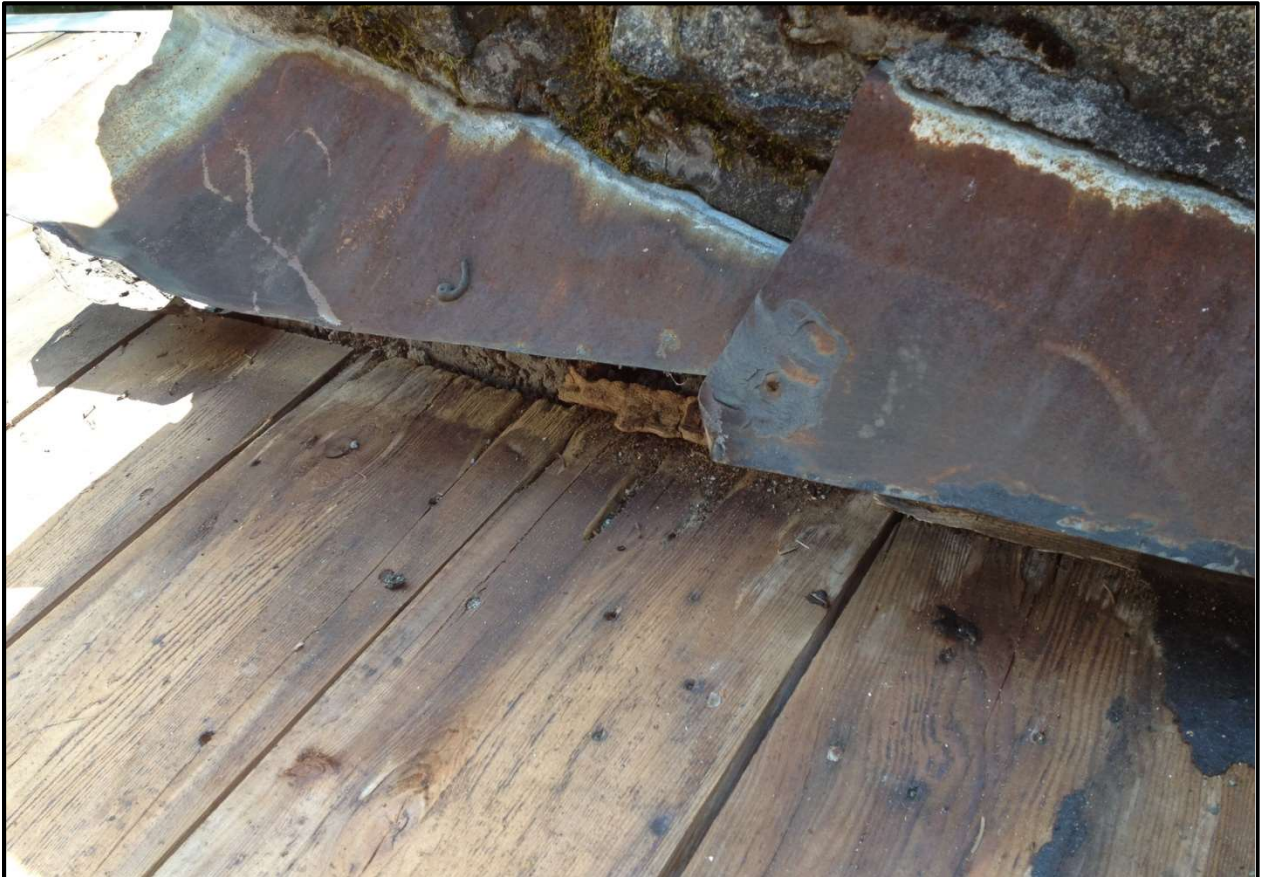
Ant nest/damage on roof at chimney interface prior to roof replacement on LH.
